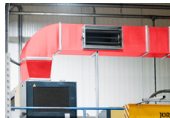
This conduit distributes the waste heat from the compressors.
